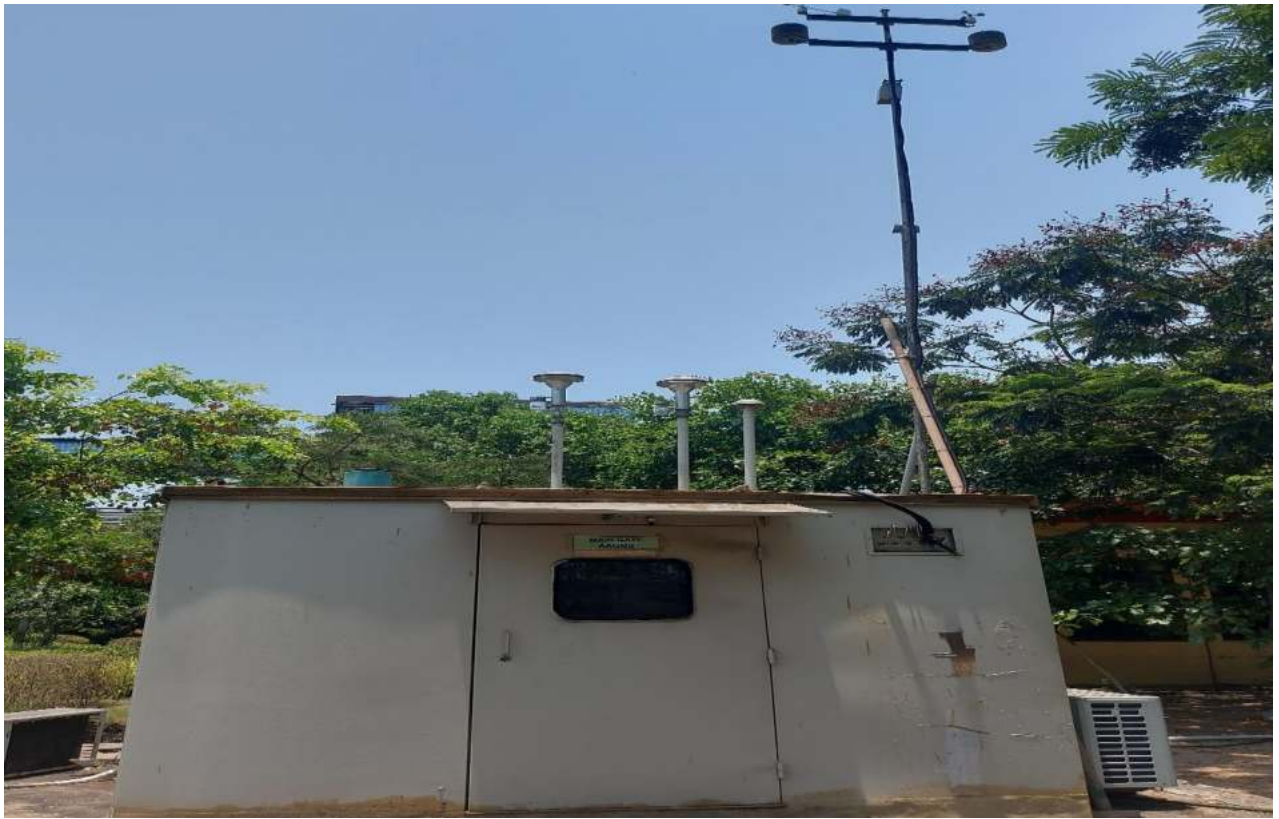
CONTINUOUS AMBIENT AIR QUALITY MONITORING STATION INSIDE THE PLANT
