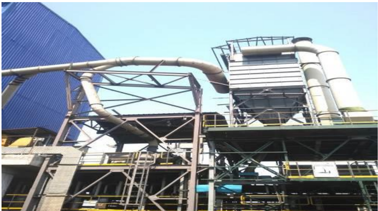
DUST EXTRACTION SYSTEM AT TRANSFER POINTS
